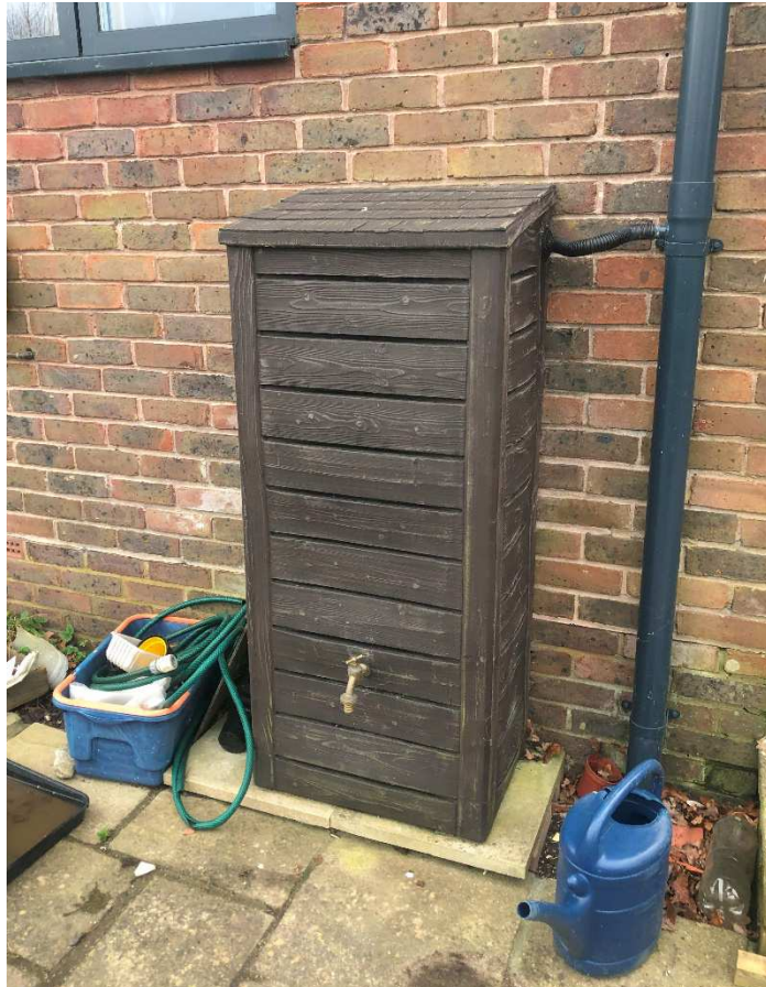
230 litres outside kitchen
