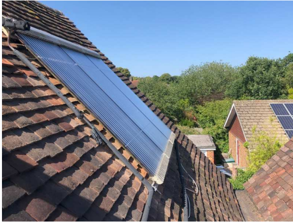
Solar thermal panel
